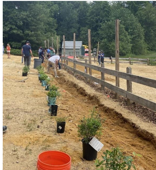
Volunteer crew helping to implement stormwater and erosion BMPs in the YMCA Camp Lincoln beach area. Photocredit: FBE
