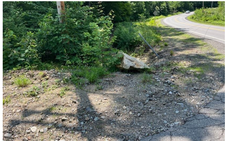
Stormwater erosion along Coburn Hill Road to the downhill side of the culvert parallel to Main Street.
