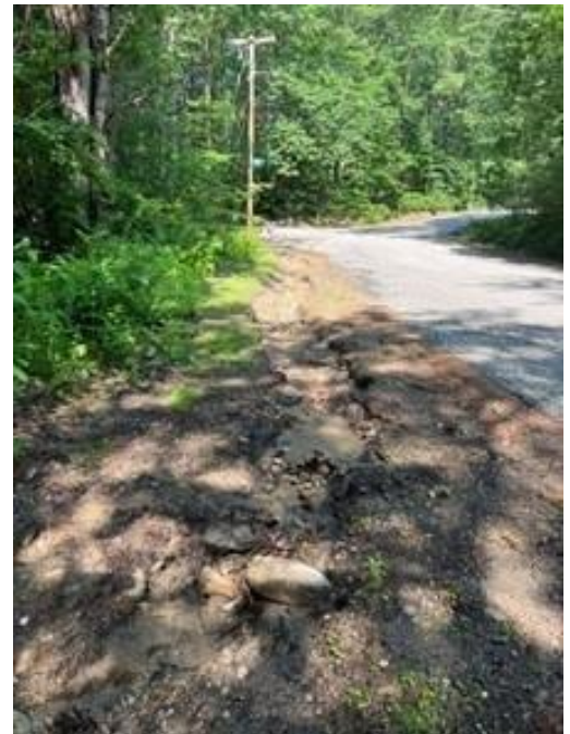
Road shoulder/ditch erosion on Long Pond Road near Pine Street, July 2023. Photo credit: FBE.
